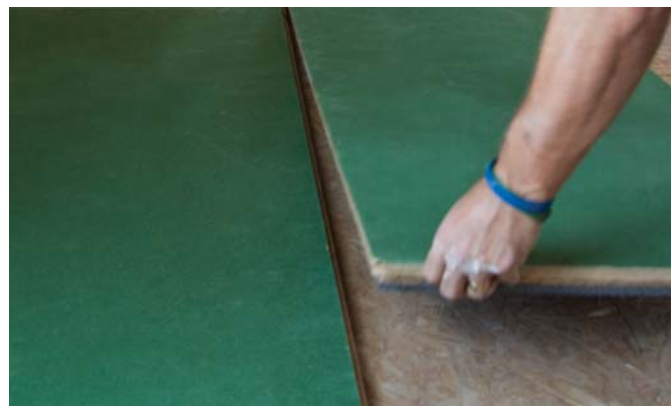
3. The board is installed tight against the edging strip, laid in a staggered pattern with no gaps between the boards.
