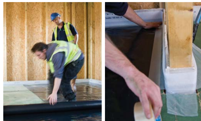
4. A slip membrane with minimum 500µm thickness is laid, lapped and taped at the edges and the laps.
