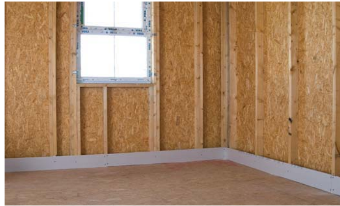
1. Installation of a 150mm plasterboard rip with 5mm gap to the structural deck, so there is a solid back for the SoundBar Gyvlon screed.
