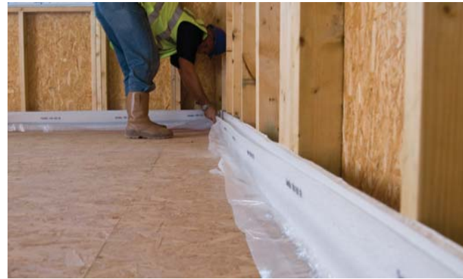
2. The SoundBar edge strip is installed with the self adhesive backing against the plasterboard rip.
